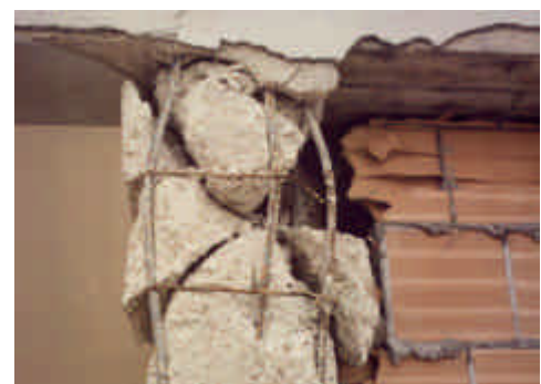
Figure 4. Damage after 2 nd shock (same column as in figure 3) (photo: A. De Sortis)
