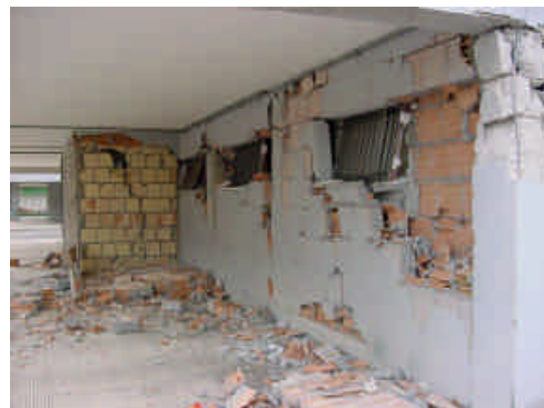
Figure 2. Damage to the columns of the 4 story building after the 2 nd shock (photo: P.Bazzurro)
