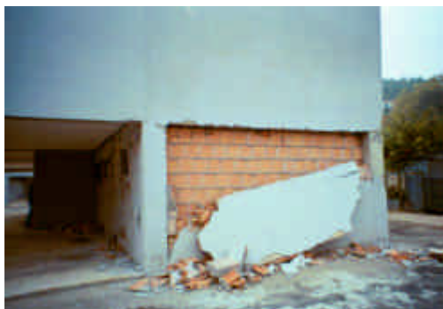
Figure 3. Damage to the 4 story building after the 1 st shock (photo: M. Mucciarelli)
